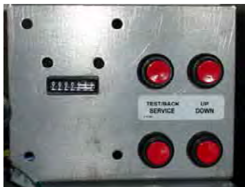
Figure 5. Operator Button Panel
