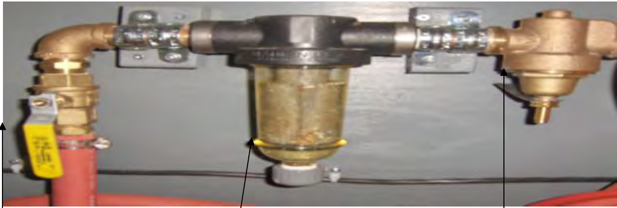
Shut off valve
